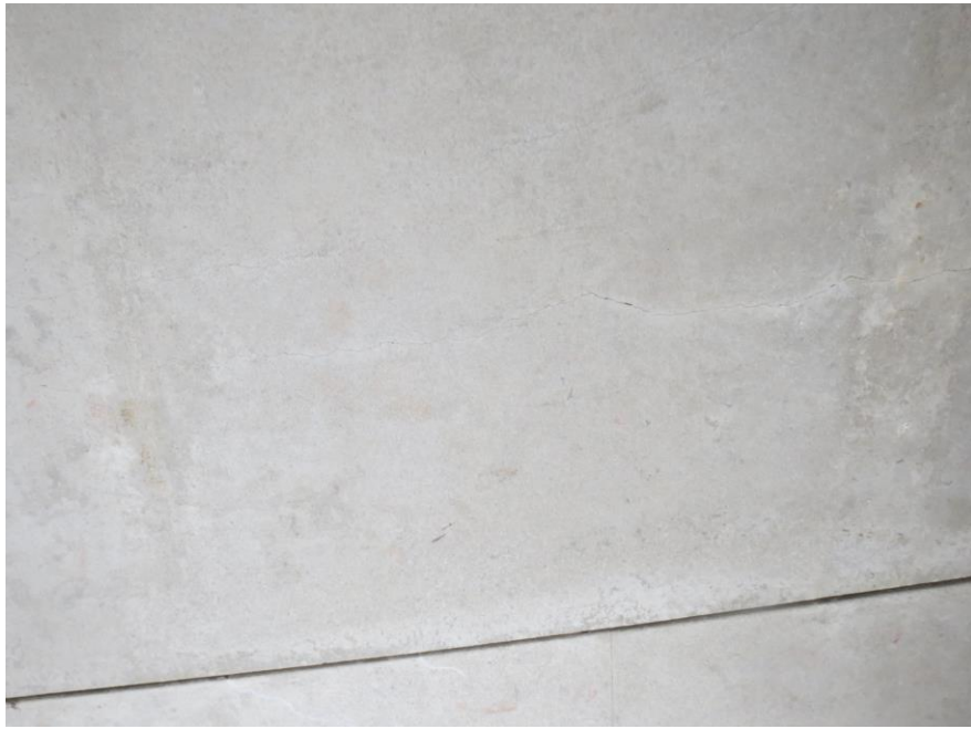
DECK PANEL BAY "B" SP. #3 W/ CRACK
