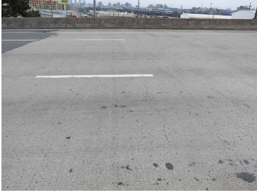
WEARING SURFACE SP. #1 W/ SCALE & CRACKS
