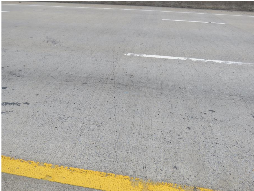
WEARING SURFACE SP. #3 W/ SCALE & CRACKS
