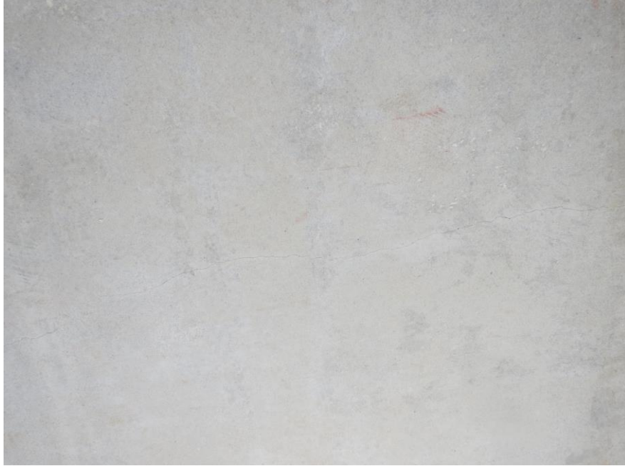
DECK PANEL BAY "A" SP. #3 W/ CRACK
