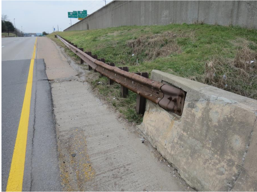
GUARDRAIL "B" END RT. W/ CORROSION
